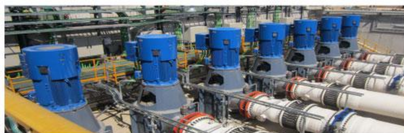
Cooling water & Water supply plants
