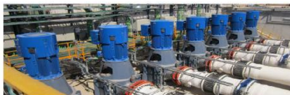
Cooling water & Water supply plants
