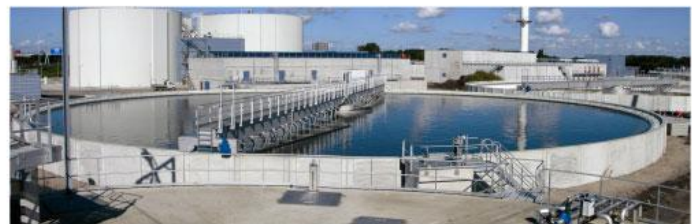
Effluent Treatment & Sewage Plants
